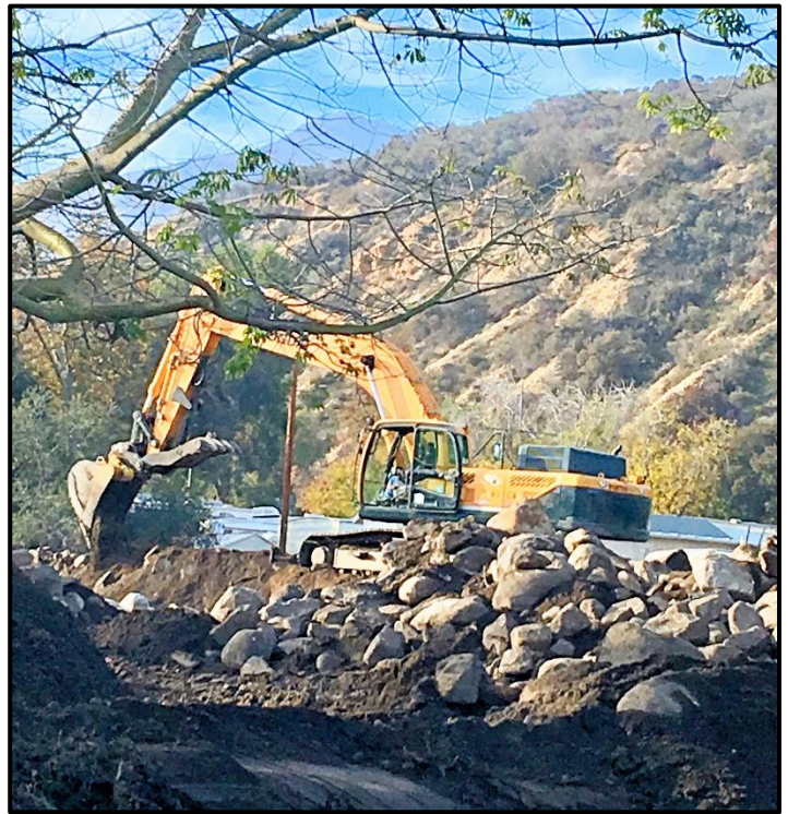
WITH A LITTLE HELP OF OUR FRIENDS: A volunteer operating rented equipment moves mud, rocks and debris at Glen Eden.
