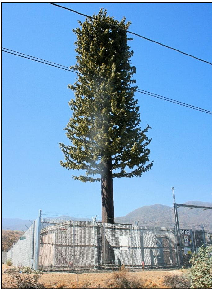
"CAN YOU HEAR ME NOW?" Verizon is counting on better service for customers with the installation of this cell tower on Temescal Canyon Road adjacent to the IvyGlen substation.
